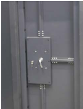
Typical high security lock detail
